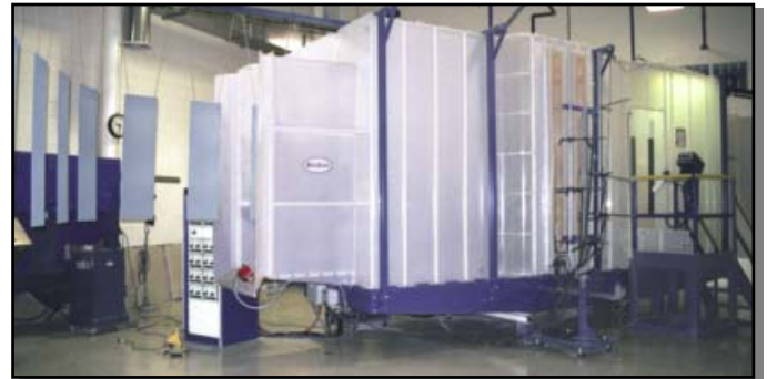
Powder paint facilities.
