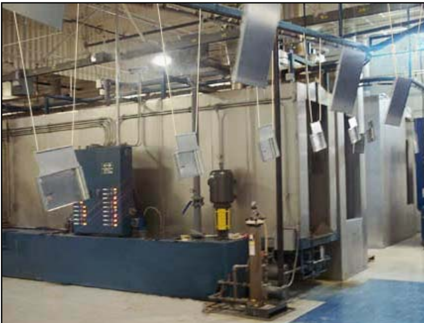
The automated wash system and dry-off oven.
